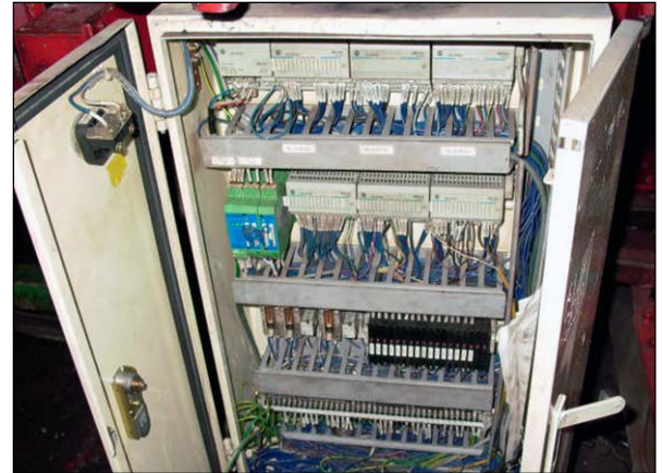
Figure 2: Cabinet mounted I/O example
